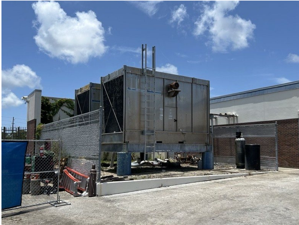
Chiller Plant Before
