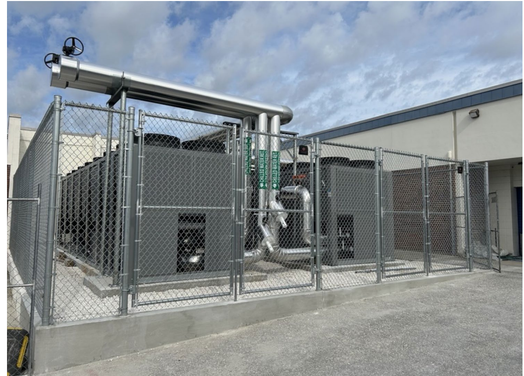
Chiller Plant After
