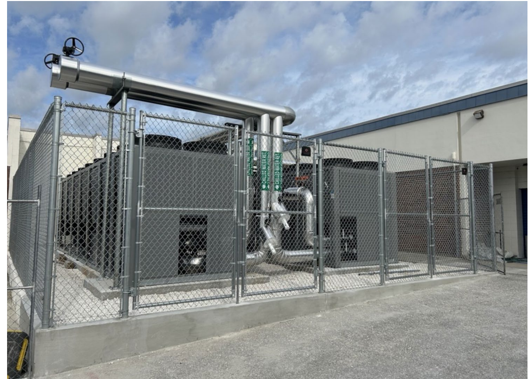
Chiller Plant After
